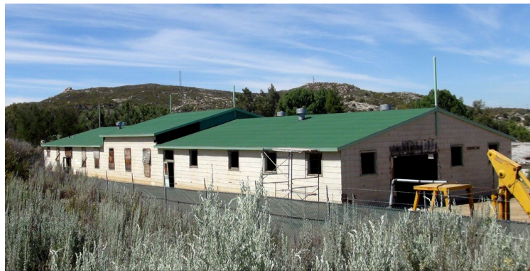
We have now completed the contractor installed roof on the first building and it looks outstanding!
